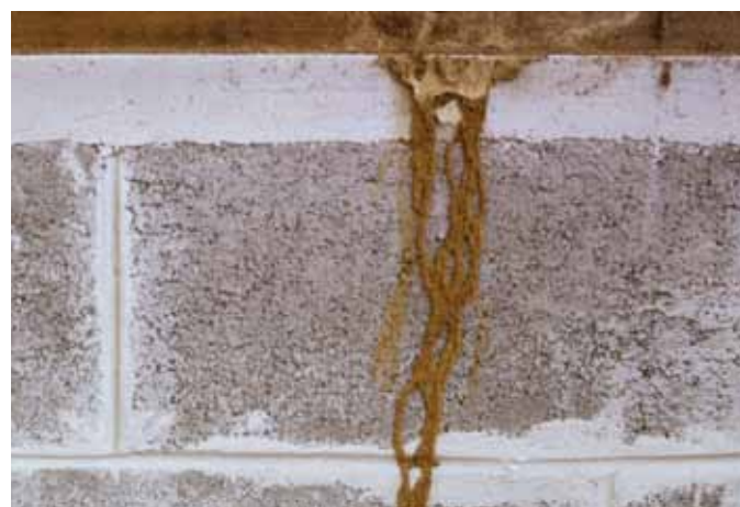
Fig. 2. Subterranean termites build protective mud tubes to prevent desiccation while foraging. 2
