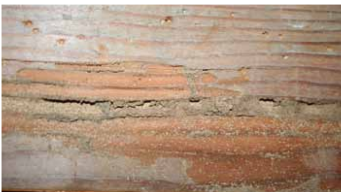
Fig. 8. Subterranean termites often feed along the spring wood and leave behind frass. 7
