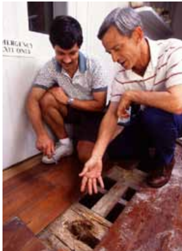
Fig. 10. Subterranean termites can shred solid wood beams. 4
